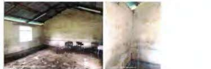
Interior of the classroom block that have been condemned; note the structural damage along the walls
