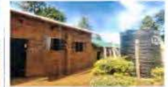
Existing dilapidated classrooms
