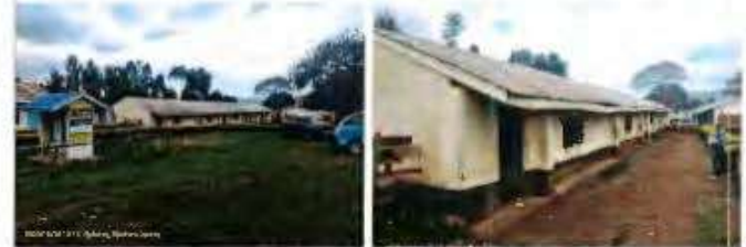
View of the 4 classroom block that has been condemned for demolition
