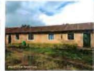
Classroom block with dilapidated roof cover
