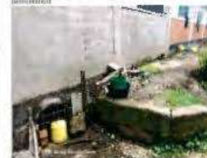
Drainage culvert between classrooms that channels storm water away from the neighbouring primary school
