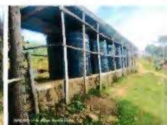
Rain water harvesting tanks, the main source of water
