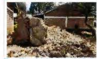
Demolition of water storage tank to allow for construction of the new laboratories
