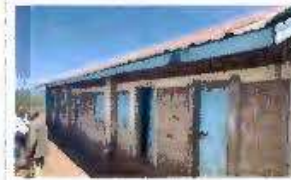
Existing dilapidated class-rooms
