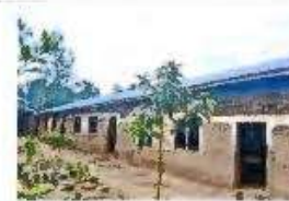
Existing in dilapidated condition
