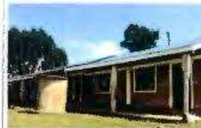
Classrooms in disintegrated condition
