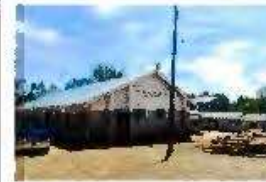
KPLC power line and switch board to be relocated
